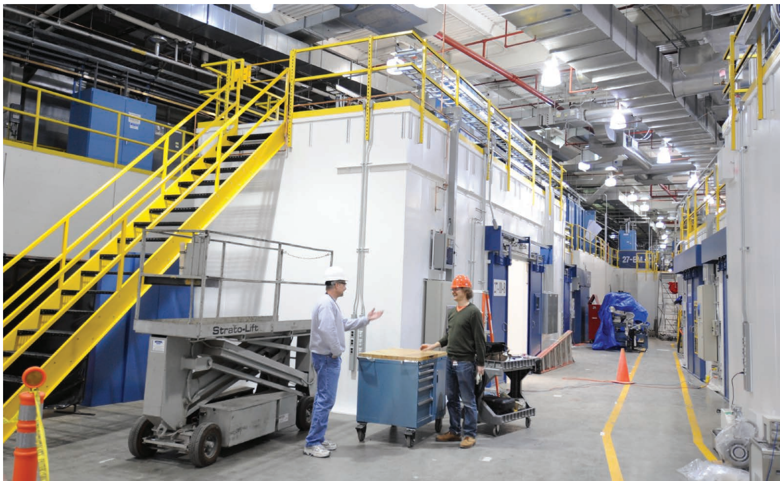
Richard Krakora (left) and Thomas Gog (both XSD) at 27-ID, under construction, April 2, 2014.
