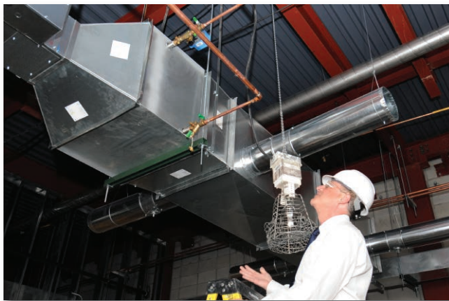
Marvin Kirshenbaum (AES) checks one of the modified high-efficiency reheat coils installed in laboratory/office module 438F at the APS.
