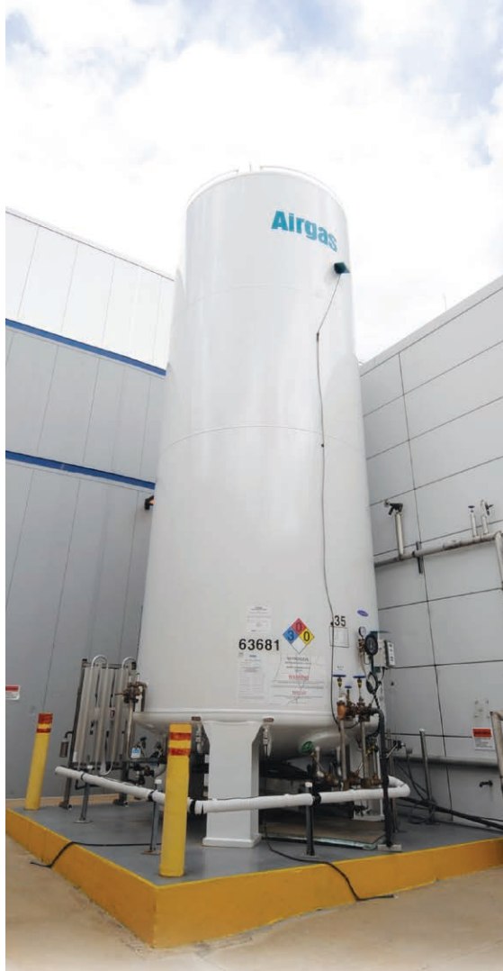
Fig. 1. One of the 9000-gal LN 2 tanks.
