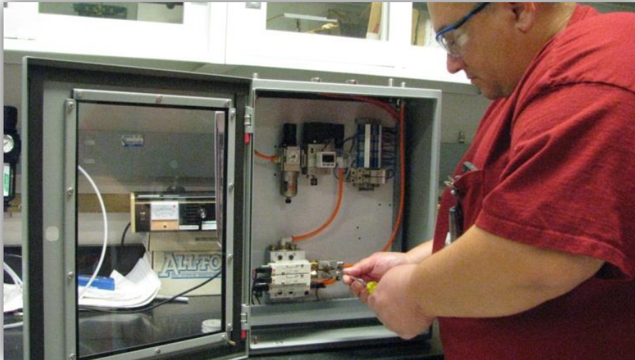
Robert Wilson - Upgraded Pneumatic Door Box
