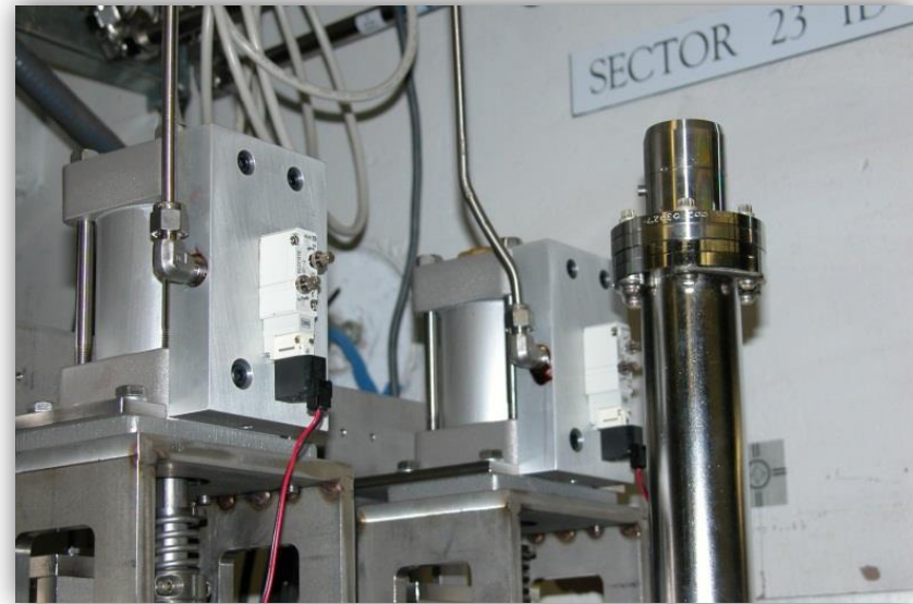
New Front End Pneumatic Cylinders at 23 ID
