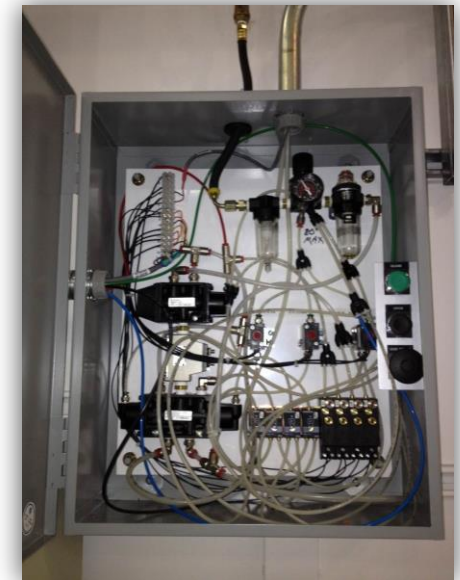
Existing Pneumatic Door Box
