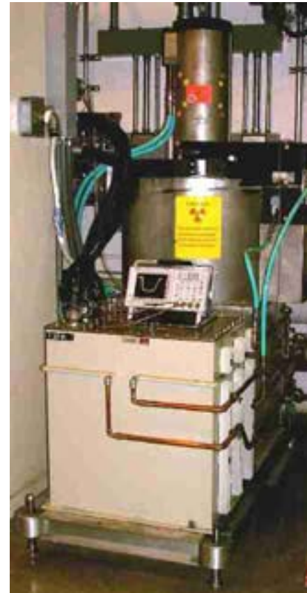
Klystron Tank Assembly
