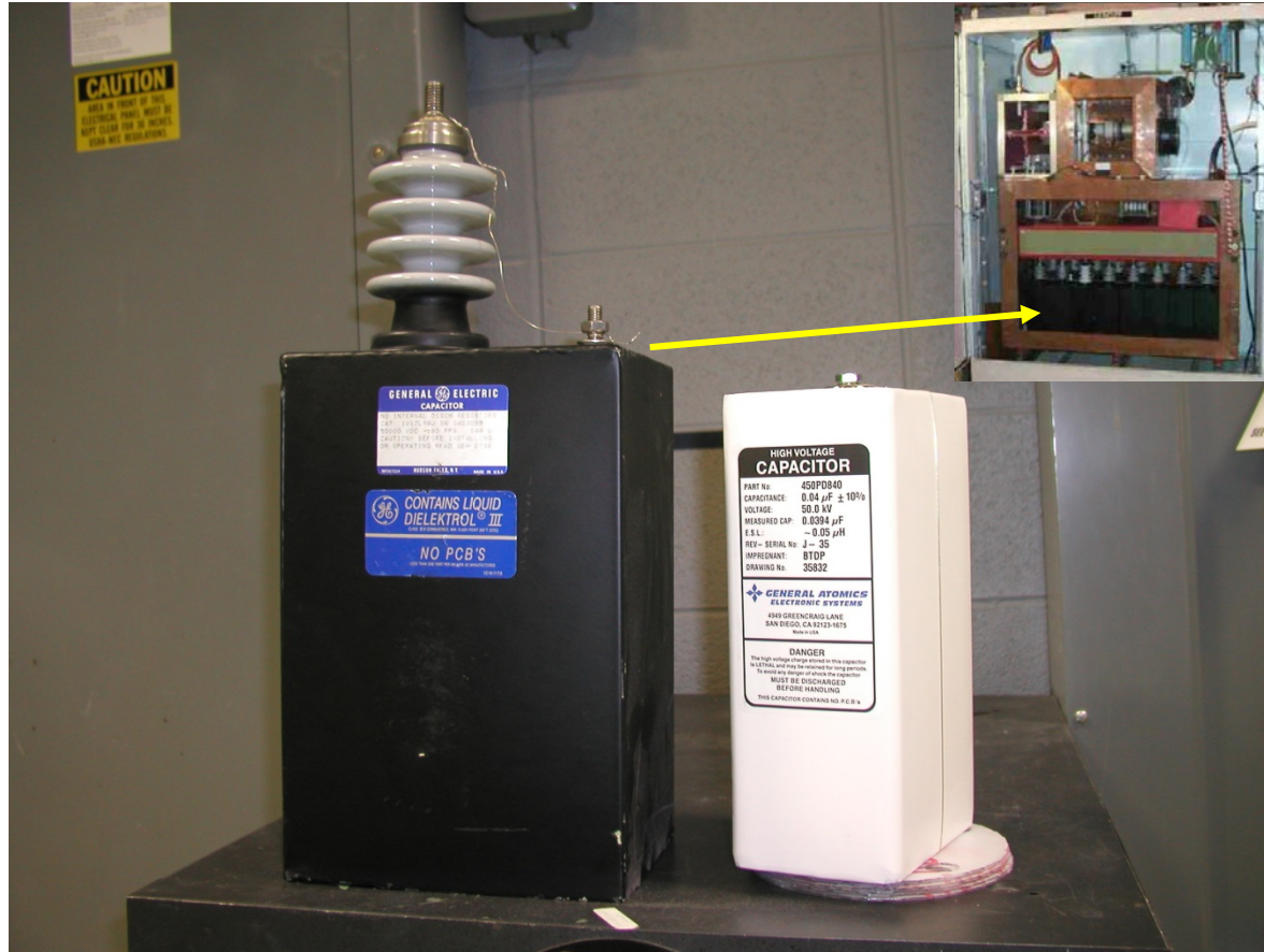
Old & New PFN Capacitor
