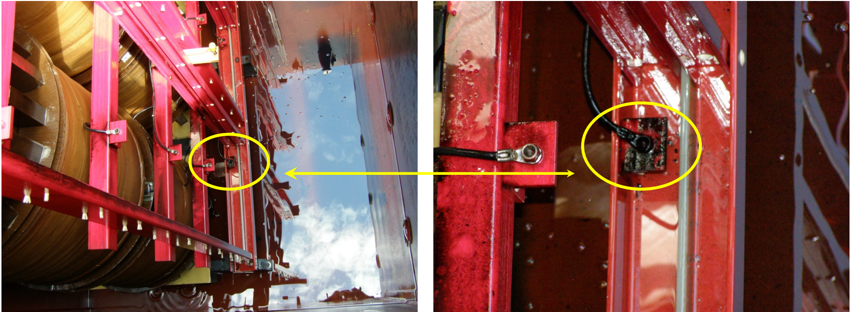
RF3 TR Set diode stack connector fault.
