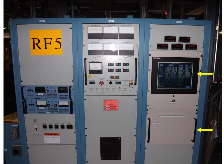
NEW PLC CONTROL SYSTEM TO REPLACE ORIGINAL OBSOLETE CONTROLS
