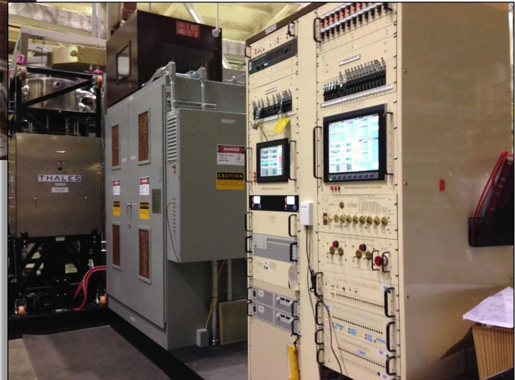
Filter Cabinet and PLC Controls
