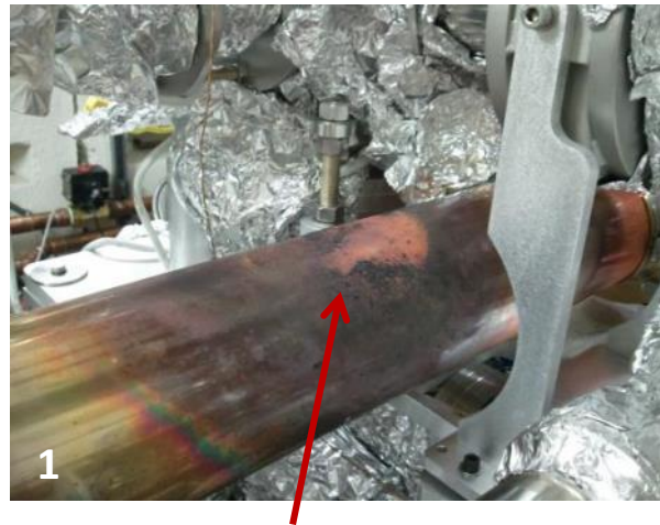
Main Overheated area
