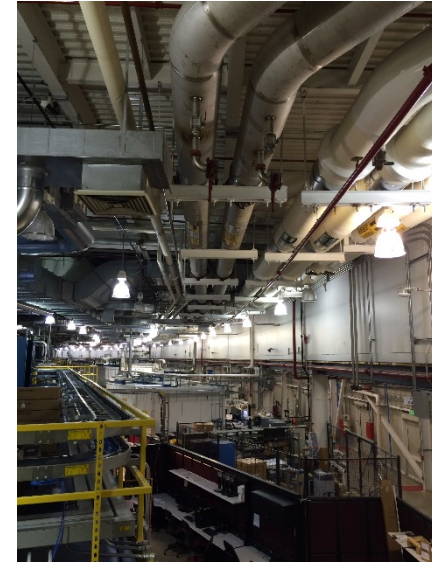
Exp Hall Primary Water Mains
