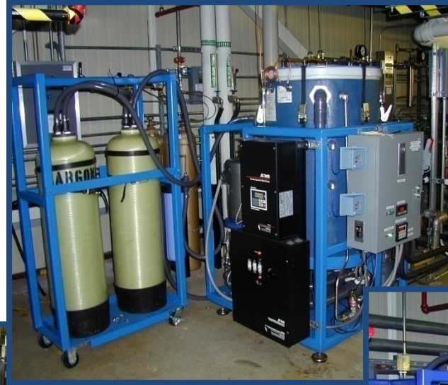
APS Designed Skid with Modifications
