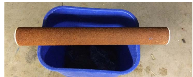
Chilled Water Filter
