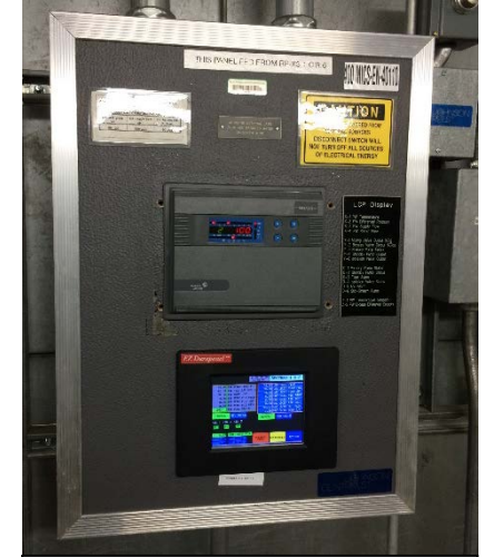
Johnson Controls Panel
