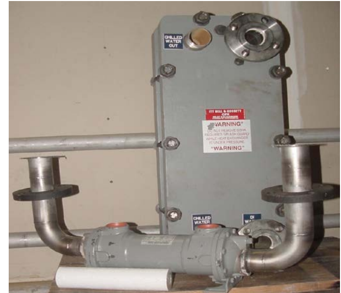
Old Plate and Frame Heat Exchanger and New Shell and Tube Type Heat Exchanger
