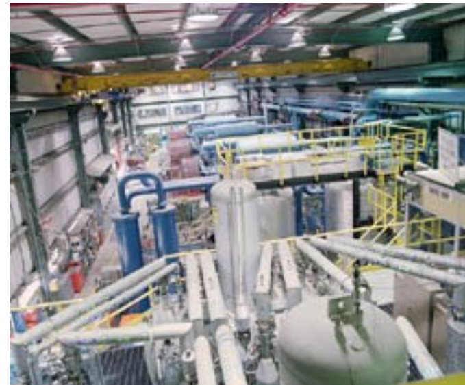
FNAL's Central Helium Liquefier. Part of their 24 kW 4.5 K helium system.
