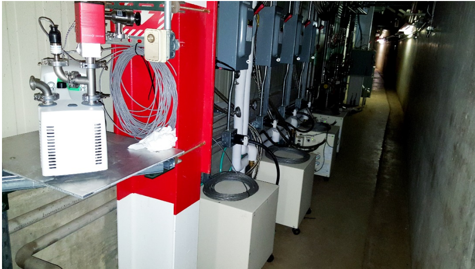
Cryocooler chillers (4) and vacuum roughing pump in utility corridor.
