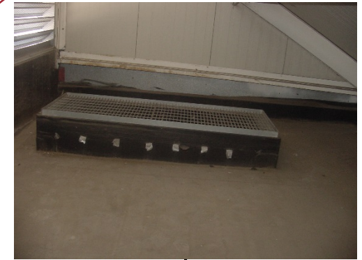
Outside Air Intakes
