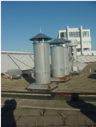
Outside Air Exhausts
