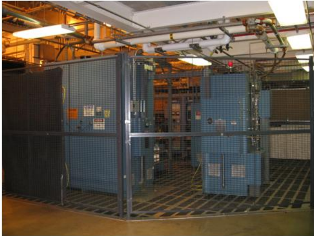
APS Booster/Storage Ring High Voltage RF Systems
