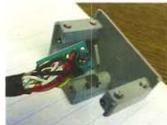
The damaged wiring insulation and carbon deposits on the metal shell cable connector.
