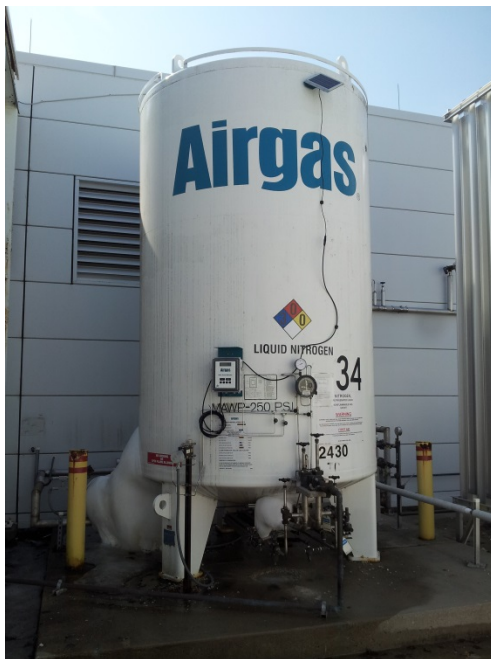
Typical 3000 Gallon tank at APS
