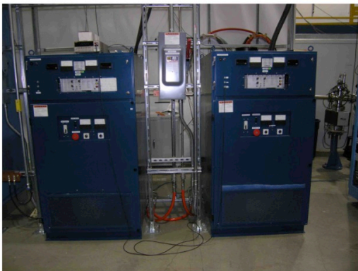
OCTUPOLE POWER SUPPLIES
