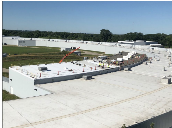
Fig. 21. Left: cover of the “Advanced Photon Source (APS) Infrastructure Master Plan Volume 1.” Right: completed replacement (400,000 ft 2 ) of the storage ring roof in 2021.
