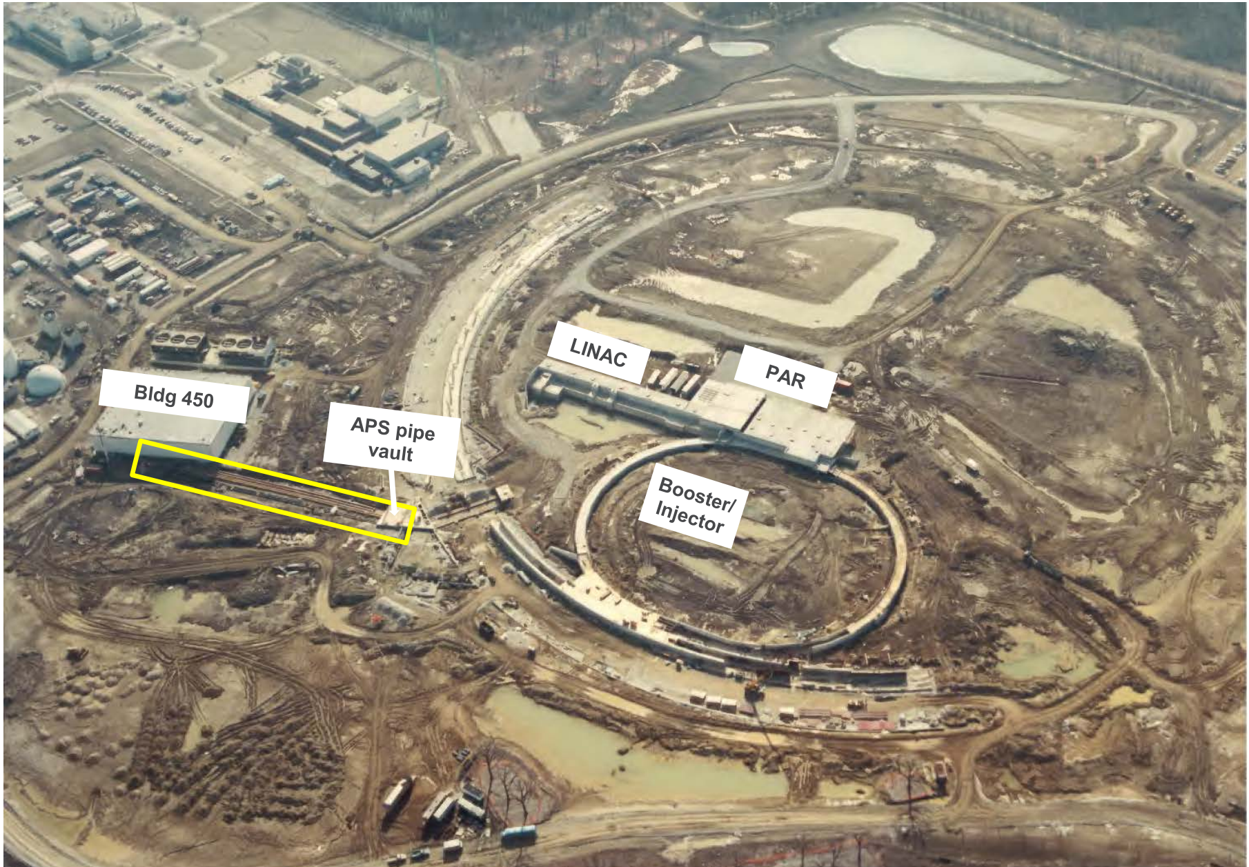
APS construction photo (undated) showing bank of piping, outlined in yellow box above, that includes the LTHW supply and return from Bldg. 450 to the APS pipe vault.
