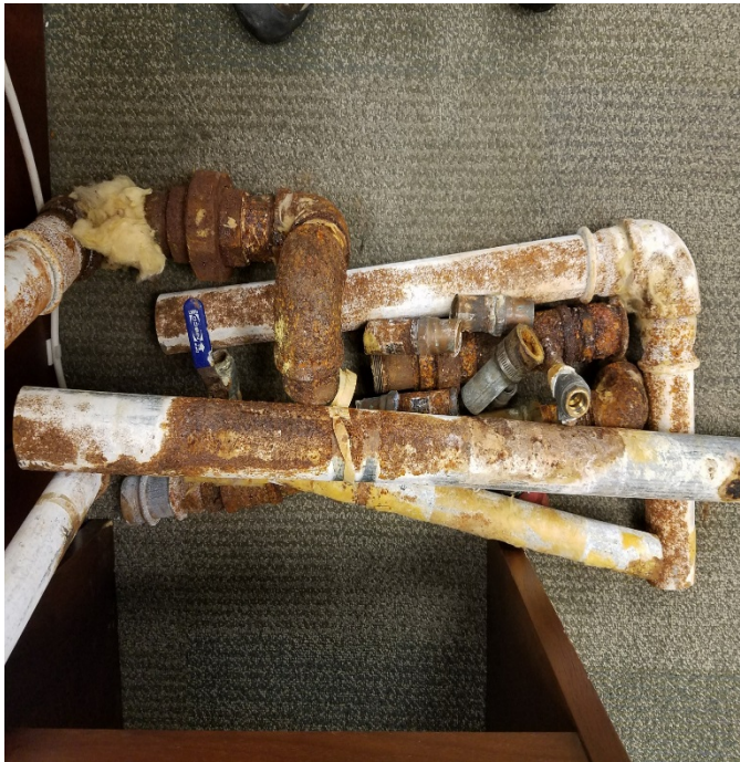
Before: Sample of removed piping shows extent of degradation
