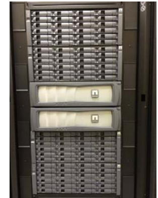
NetApp FAS-8040 Storage System
