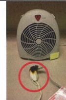
Heater plugged into extension cord
