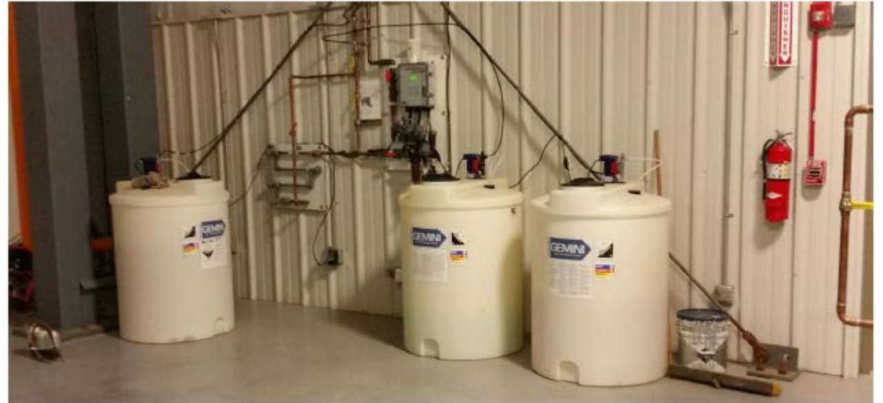
Sample Water Treatment Station, not showing Lab Sink
