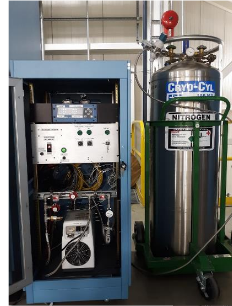
Nitrogen source and control cabinet located on SR mezzanine (left)
