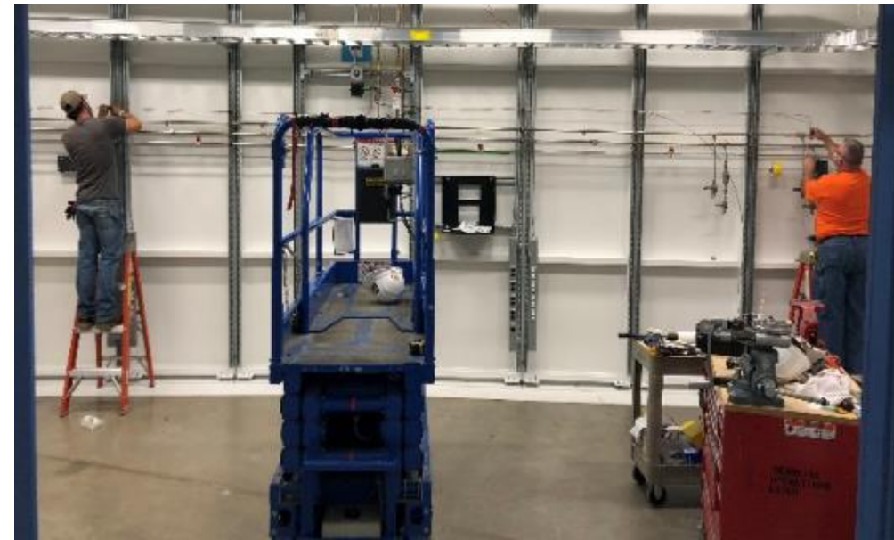
Air and water installation at 28-ID B-hutch
