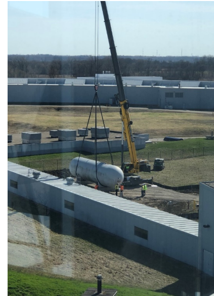
Helium tank installation for bunch-lengthening system
