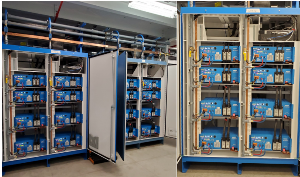
Unipolar power supply converter cabinets and the units under test in elevated-temperature room
