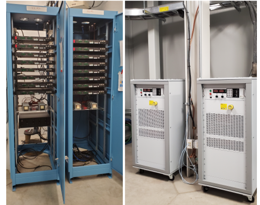
Bipolar relay rack loaded with 16 bipolar power supplies, and the raw power supplies installed in elevated-temperature testing room.
