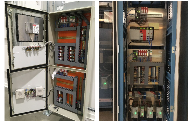
Above: 25-ID PSS controls and cabinets installed
