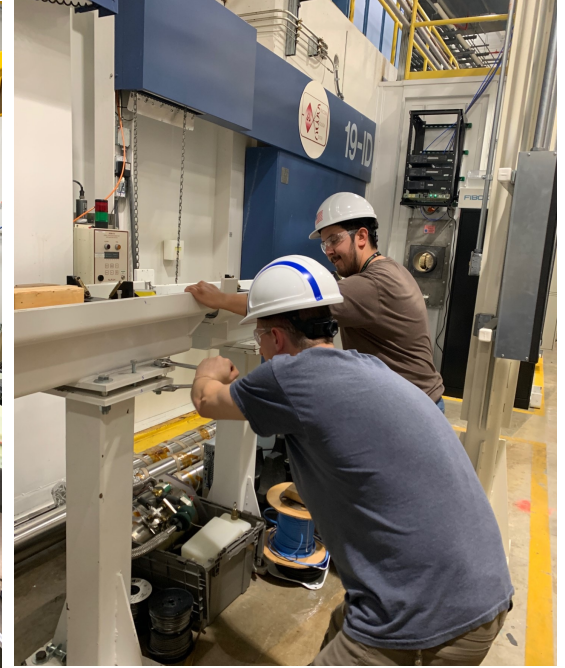
Removing sections of shielded transport to enable access into the storage ring tunnel
