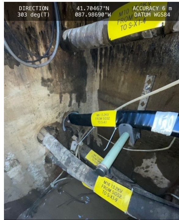
M-6 in MH-3 and cable labeling
